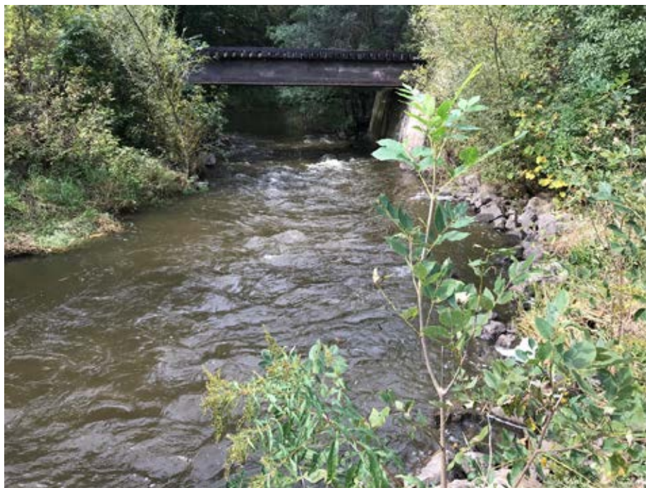
Photo 32-8 Looking upstream under a railroad bridge on the reach 4 project of Wedge Creek. Riprap was placed under bridge to control grade. Wedge creek turns 90 degrees to the left of the photo so riprap toe was installed to deflect the flow and prevent scour of the bank. State Highway 13 is immediately behind the viewer. (Wedge Creek – Reach 4, photo taken by Lucius Jonett during site visit 09/20/2019).
