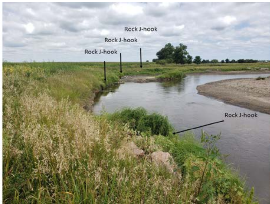
Photo 28-1. Looking upstream at the upstream project area. Locations of four of the six rock J-hook vanes are identified. Vegetation along the bank is 3 to 4 feet tall and well-established. (Photo taken 8/22/19 by Mark Prankus, Cardno).
