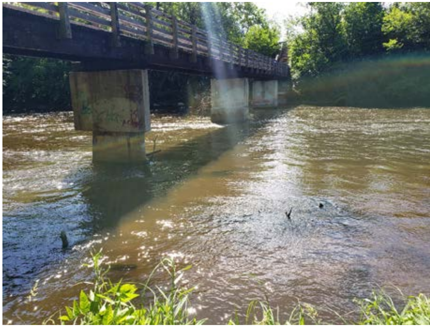
Photo 30-5. Looking at the form location of the low head dam at the top of the project. The dam was higher through the middle section than on the sides pushing water against the bank on the downstream end. (Photo taken 6/26/19 by Mark Prankus, Cardno).
