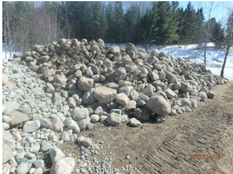
Photo 26-2. Example of the stone material installed at the County Rd 98 riffle location in 2018. Material is similar to what is naturally found in the adjacent areas of the Rat Root River. Photo provided by Koochiching County SWCD.
