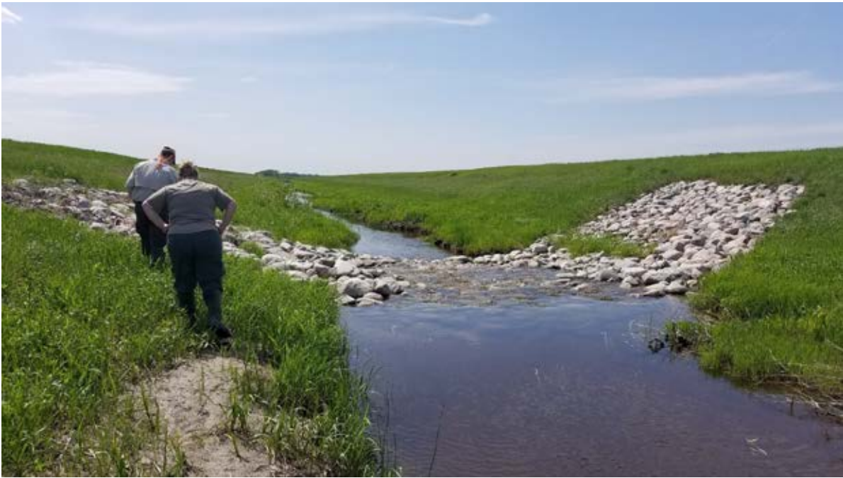
Photo 14-5 Upstream view of riffle #8. Creek is 1-2 channel widths upstream (front) and 2-5 channel widths downstream (back). This riffle is meeting project goals of reducing bank erosion. Photo taken by Ed Matthiesen during site visit (6/4/19).
