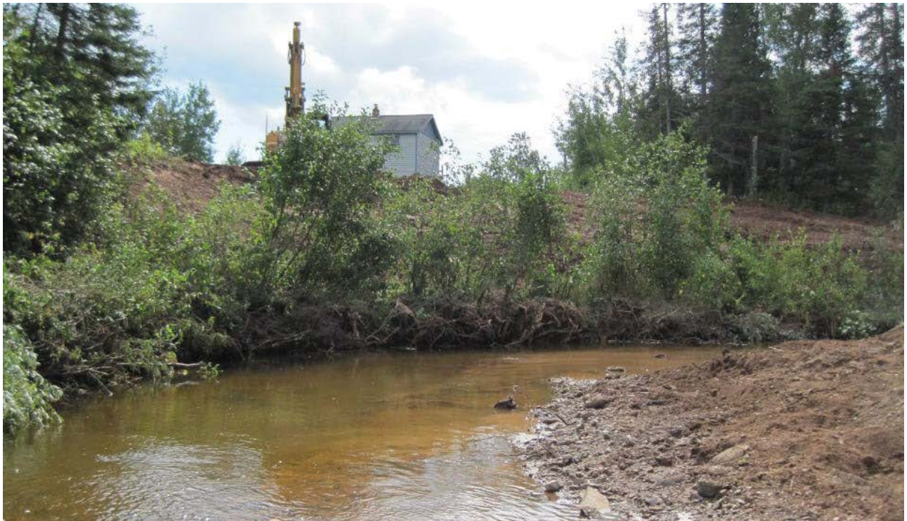
Photo 4-6 Toewood completed 09/13/2011. Top layer of toewood is live sod mats from nearby patches of Willow, Dogwood and Alder. Photo South St Louis SWCD.
