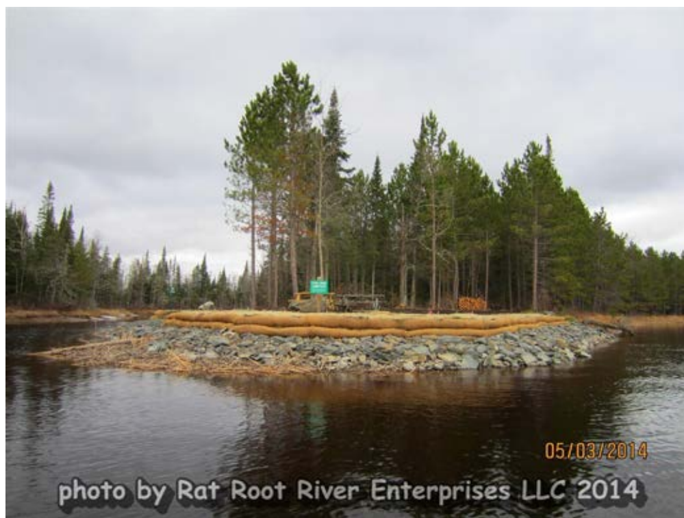
Photo 25-2. Example of the Fish Camp bank stabilization site in spring 2014 following construction in fall 2013. Photo provided by Ed Lombard, Rat Root River Enterprises, LLC.
