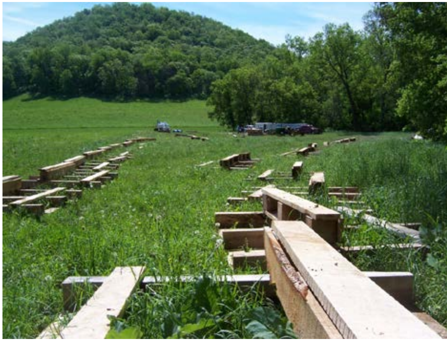
Photo 22-7. Example of Minnesota sky hook structure. The structure provides overhead cover for fish. It is assembled in the dry and placed into the bank. Photo taken August 2011 and provided by MN DNR.
