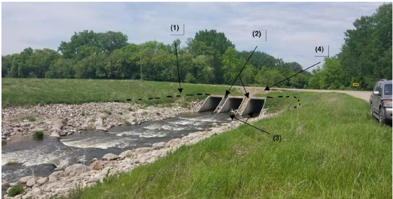
Photo 16-12 Sand Hill River fishway ramp #4. This area of the project has experienced some changes after high flows in spring 2019 came up over the road. Further damage could be mitigated by adding riprap of the same size to the top of the culvert on both sides (1) hand-placing riprap between culverts (2) and repairing the slop with topsoil/seed/25 blanket (4). Project partners also discussed considering rock or a barrier to force low flow into one box. Photo taken by Ed Matthiesen during site visit (6/4/2019).
