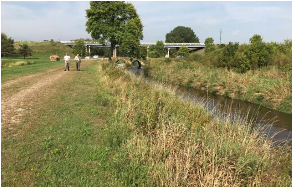
Photo 32-2 Photo looking upstream at the 12' replacement culverts. Straightened channel is typical of what is found upstream in the agriculture landscape. (Wedge Creek – Reach 6, photo taken by Lucius Jonett during site visit 09/20/2019).
