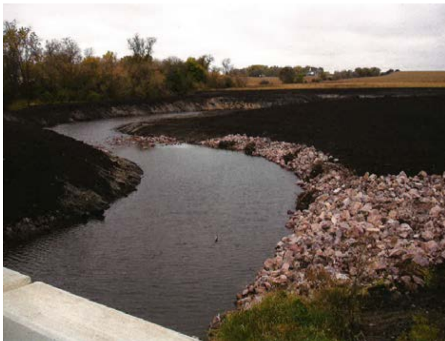
Photo 3-1 View of Elm Creek project from County Highway 36 bridge after construction and before vegetation establishment. Site evaluator questions the intended effect of rootwad placement in riprap and the elevation that the rootwads were installed. Photo taken during construction (2014).
