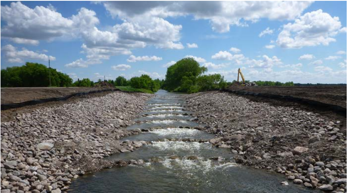
Photo 16-4 Photo of drop structure 4 after construction of fishway. Photo provided by project partners (taken 5/26/2017)
