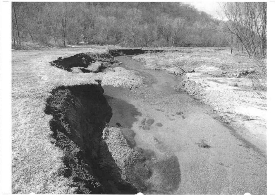
Photo 33-1 Stream conditions pre-construction. High vertical banks and overly wide stream with reduced instream habitat.
