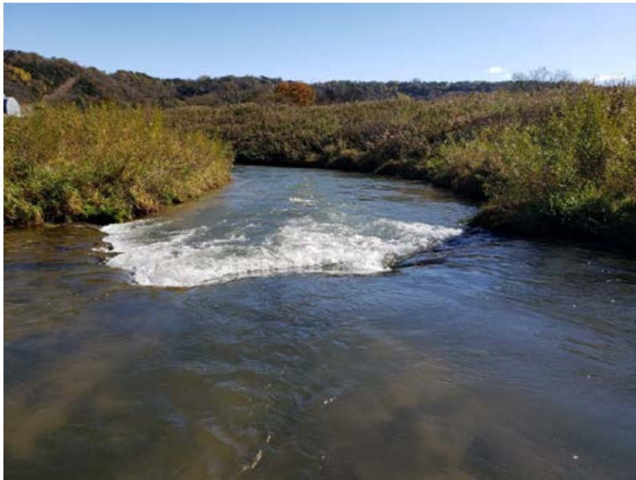
Photo 29-9 Example of one of the cross vanes installed for the project creating and maintaining a scour pool for fish habitat and energy dissipation. Photo taken on 10/18/19 by Mark Pranckus, Cardno.
