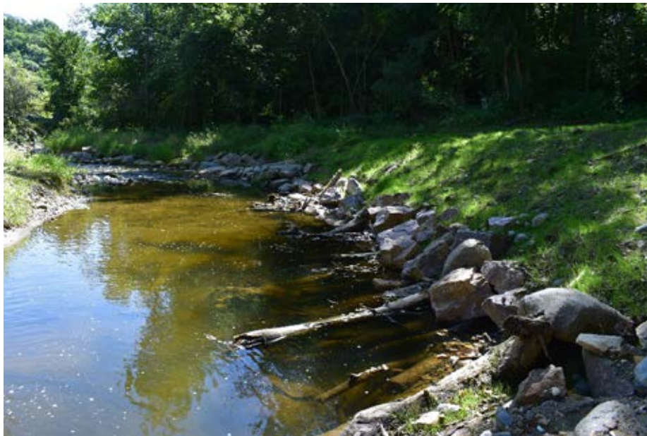
Photo 31-8 Cribwall bank after reconfiguration from parallel to streambank to perpendicular and placement of additional stone for ballast during final stream maintenance activities in August 2019. (Seven Mile Creek County Park, photo taken during site visit 08/30/2019).
