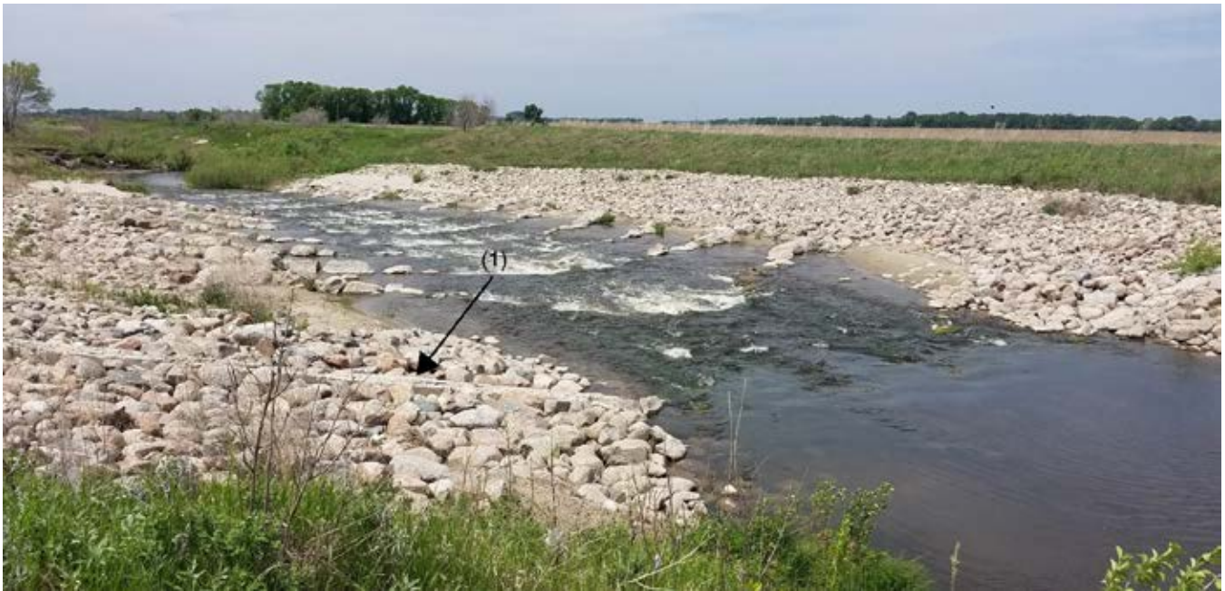
Photo 16-5 Sand Hill River fishway ramp #1 after the original drop structure was modified for fish passage. Note the cut-off weir/sheet pile in the foreground (1). Photo taken by Ed Matthiesen during site visit (6/4/2019).
