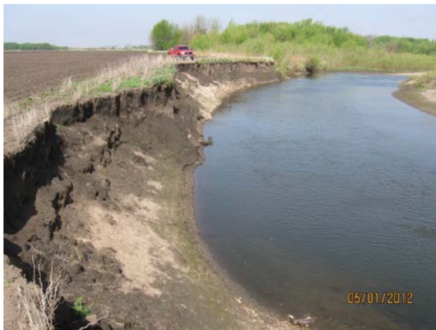
Photo 27-2. Looking upstream at the Upstream Bank (Bank 1) in 2012. In 2014, a significant flood event caused additional bank erosion prior to construction of the project (Photo provided by Scott Ralston, USFWS).
