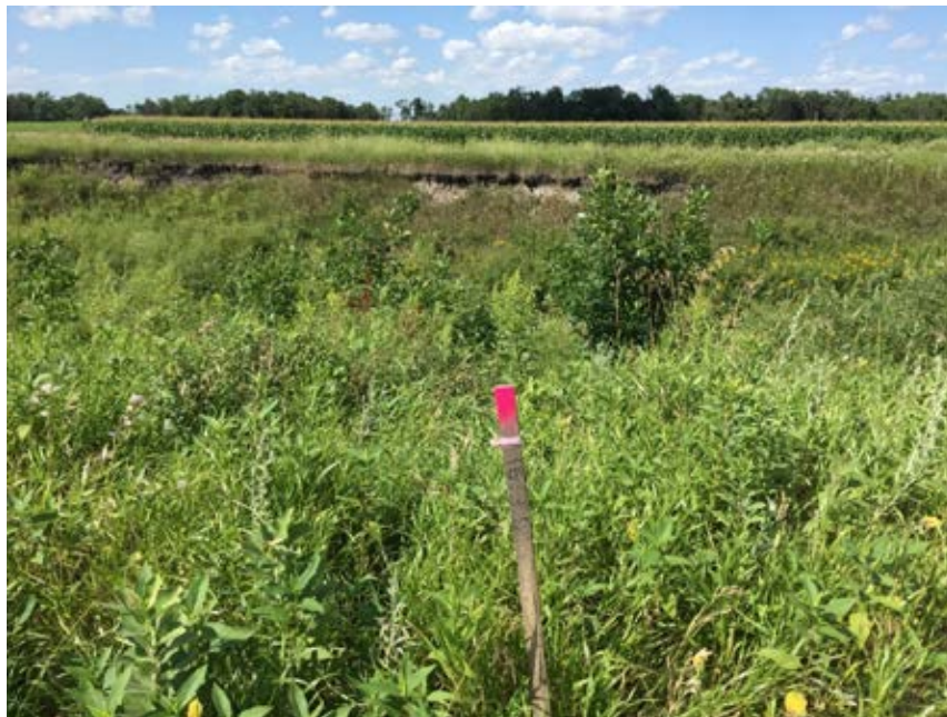
Photo 15-1 View of existing bank slump failure at project Station 91+85. Photo taken by others during pre-construction visit (8/2/2016).
