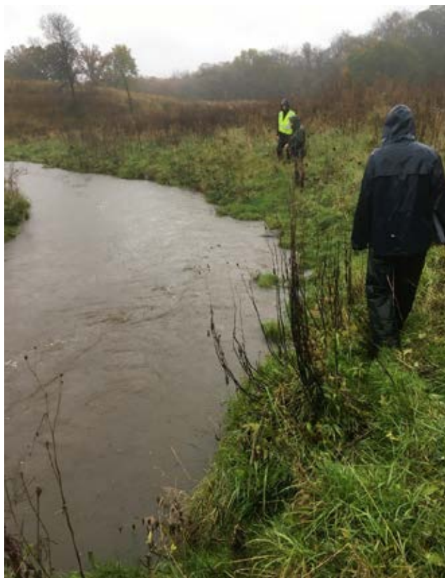
Photo 35-2 Crow Springs project area where stream bank slopes were re-shaped, and rock added. Photo taken 10/21/2019 by Anna Varian.
