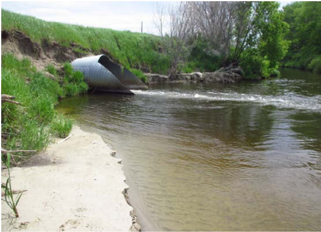
Photo 16-13 Perched culvert with erosion upstream of structure #4. Funds remaining because fishway work was completed under budget will be used to address fish passage and habitat work in this reach. Photo taken during site visit (6/4/2019).
