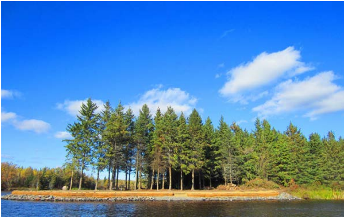
Photo 25-5. Example of the Picnic Site bank stabilization site following construction in fall 2013. Photo provided by Ed Lombard, Rat Root River Enterprises, LLC.
