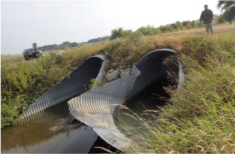
Photo 32-1 These two 12' culverts were installed on the upstream end of the project, on the upstream end of Reach 6, to replace an existing culvert that was undersized. Both culverts were incorrectly installed with an upstream invert 1.7' higher than specified. Spring runoff and ice flow in 2019 pushed up and bent the upstream end of one culvert making it non-functional. (Wedge Creek – Reach 6, photo taken by Lucius Jonett during site visit 09/20/2019).
