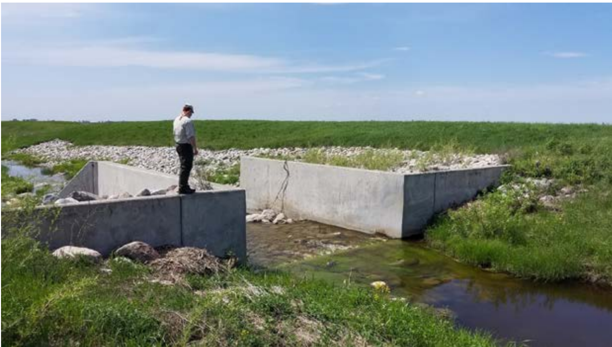
Photo 14-6 Upstream view of NRCS Rock Flume at project location 1502+00 on Burnham Creek. It is recommended to reduce the rise of the structure to less than 12 inches. Photo taken by Ed Matthiesen during site visit (6/4/19).
