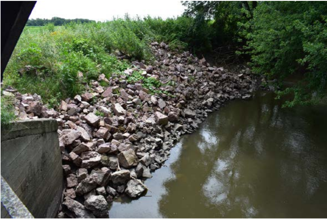
Photo 2-5 View of Adams near Bridge. Riprap protection bank. Photo taken by Ed Matthiesen during site visit (8/13/19).
