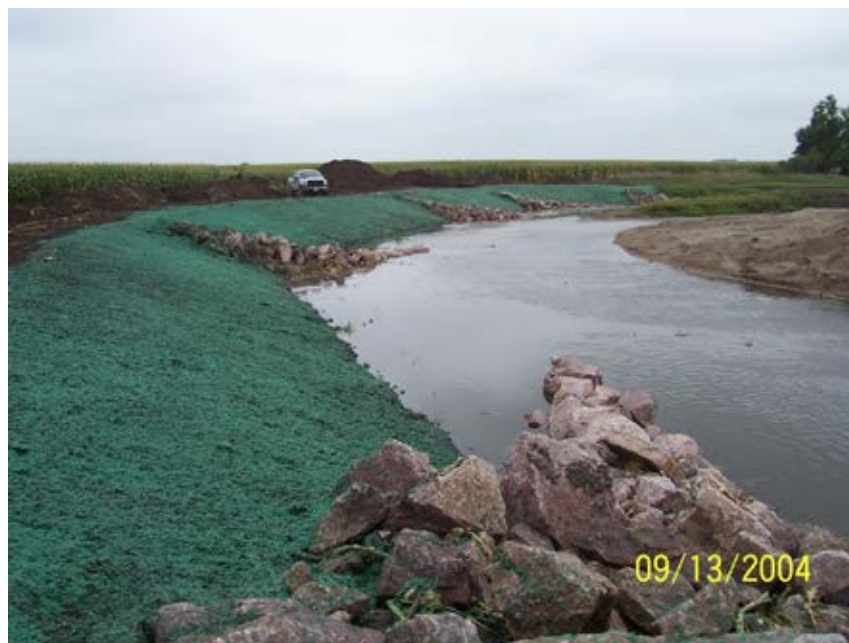
Photo 28-2. Looking upstream at the upstream project area following construction in 2014 showing five of the six rock J-hook vanes. The areas between the vanes were graded to a 3:1 slope hydroseeded with native seed mix. Notice when compared to Photo 28-1, the elevation of rock on several structures have decreased, potentially due to rock moving during high flows. Photo provided by Scott Ralston (USFWS)
