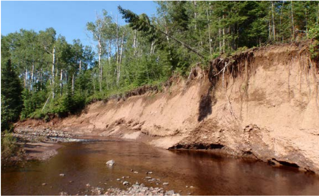
Photo 9-1 Eroding bank in the project reach June 2012 prior to 2015 project construction.
