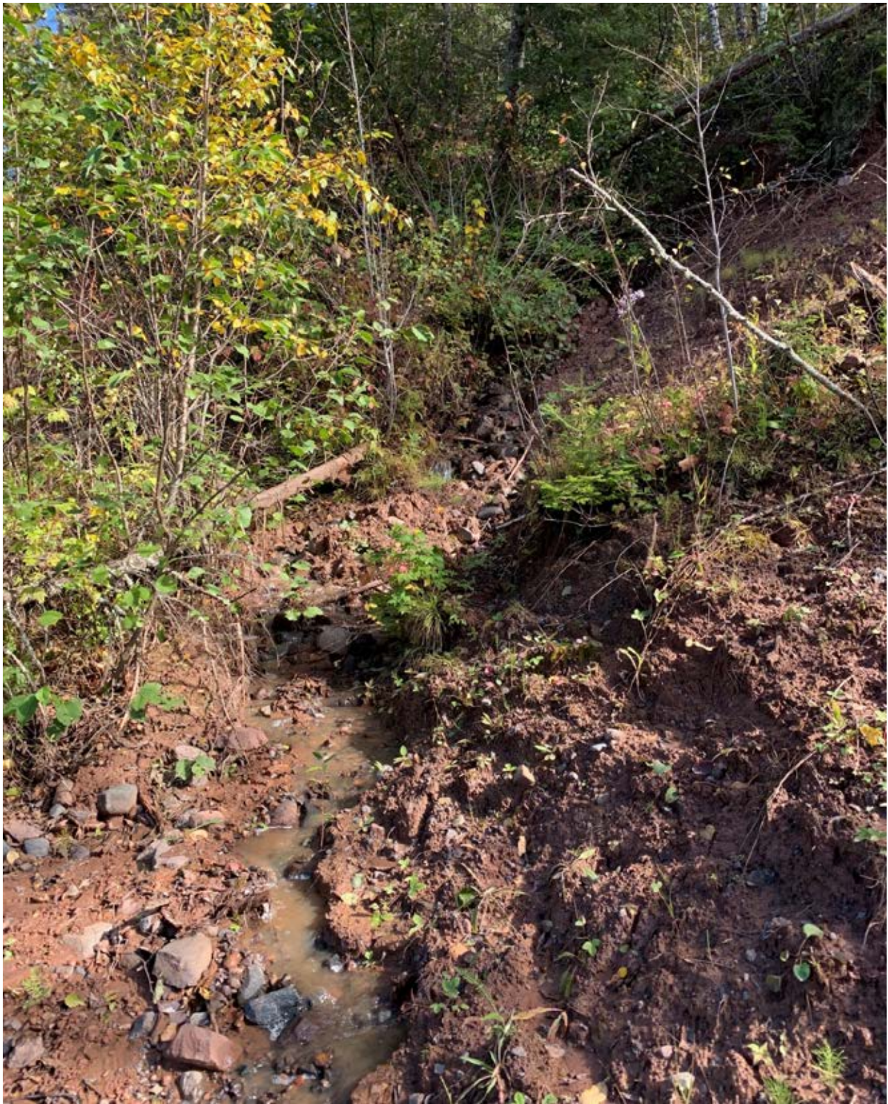
Photo 5-5 Representative image of concentrated runoff within the project reach following a previous day storm, which is yielding sediment to the Knife River. Photograph taken by Kevin Biehn on 10/1/2019 site visit.
