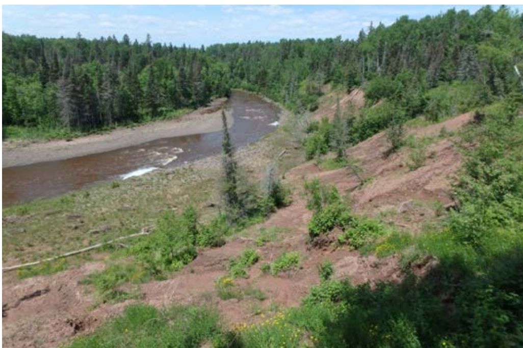
Photo 5-2 View of the project site with installed bankfull bench, July 10, 2018, two and a half years after installation.
