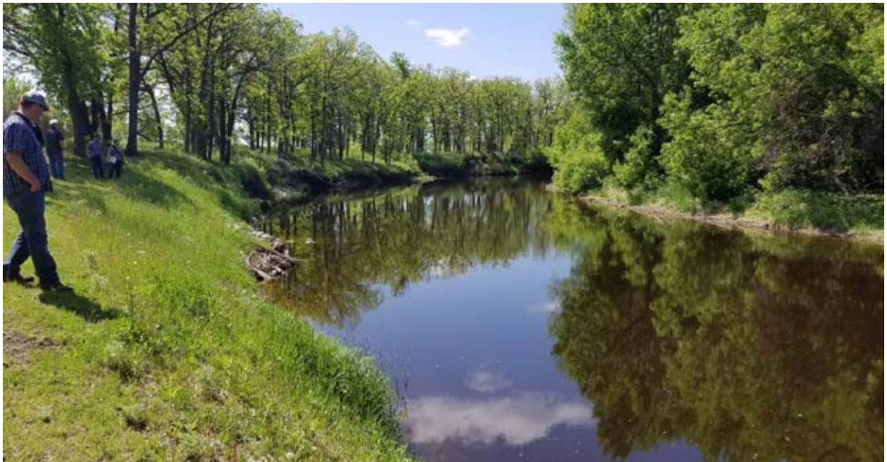
Photo 11-4 Upstream view of stream barbs 4 and 5. Mowing to the top of the bank and bare soil can be seen on the left side of the photo. Photo taken by Ed Matthiesen during site visit (6/5/2019).
