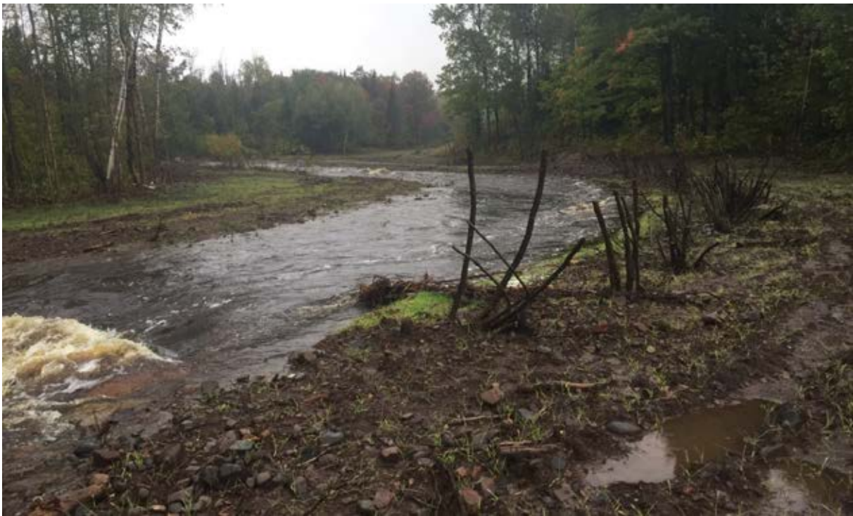
Photo 9-9 Representative image of project elements: Toe Wood (right) with willow harvested mats above and Log J Hook with Rootwad downstream (left) 09/24/2015.
