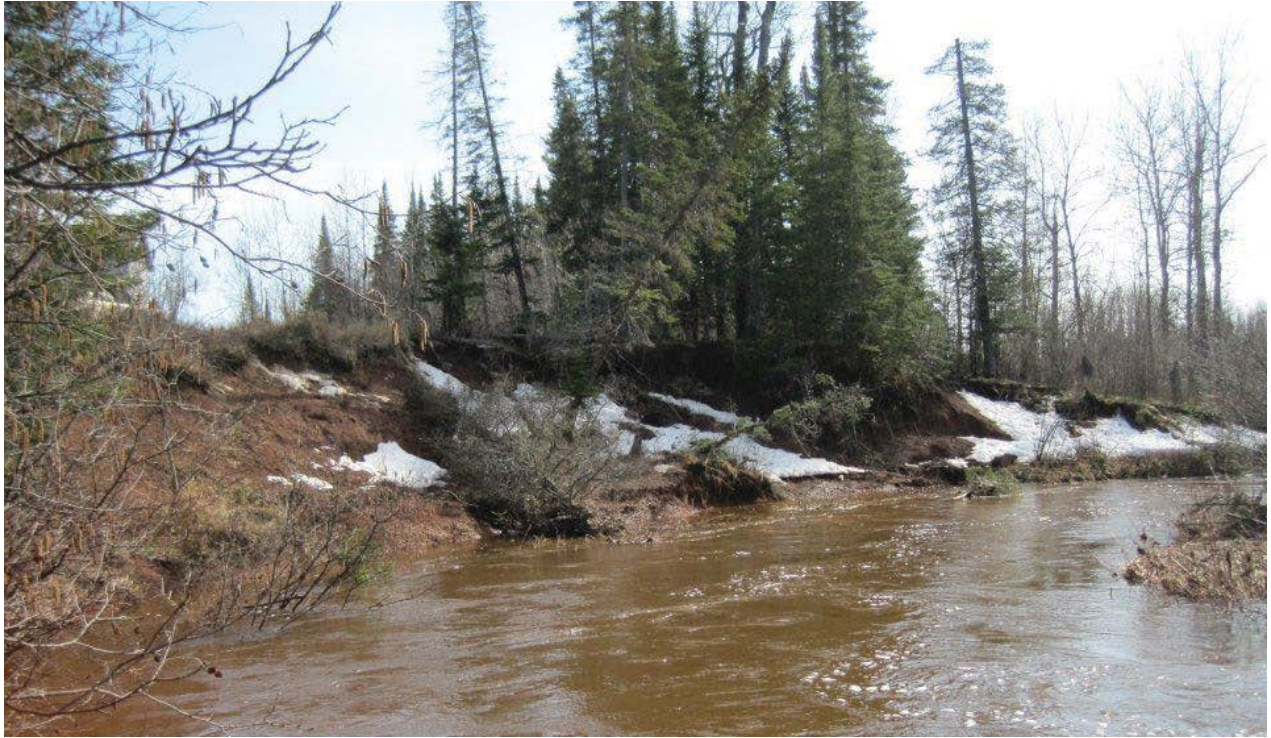
Photo 4-5 Eroding bank 04/12/2011 increasing sediment load and threatening access road and structure above. Photo South St Louis SWCD.
