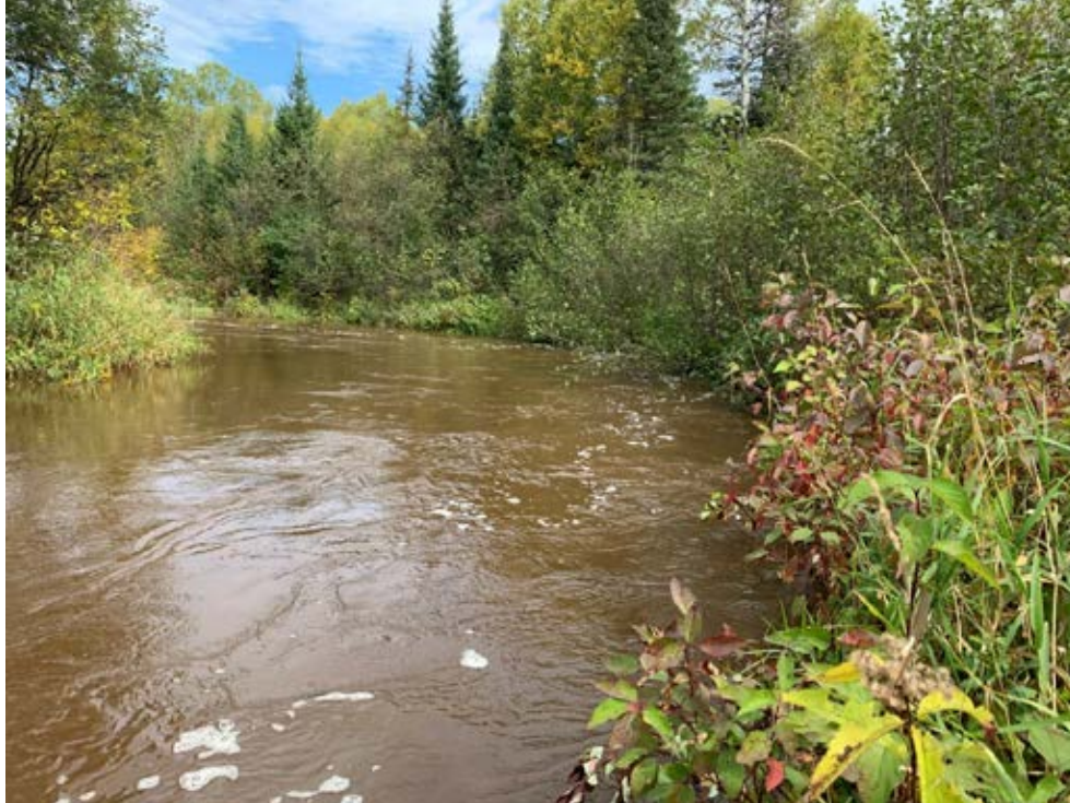
Photo 4-2 Representative image of Toewood stabilization. Photograph taken looking upstream at a period of high (near bankfull) river stage; Toewood installation is on right stream bank. Photograph taken by Kevin Biehn during 10/1/2019 site visit.
