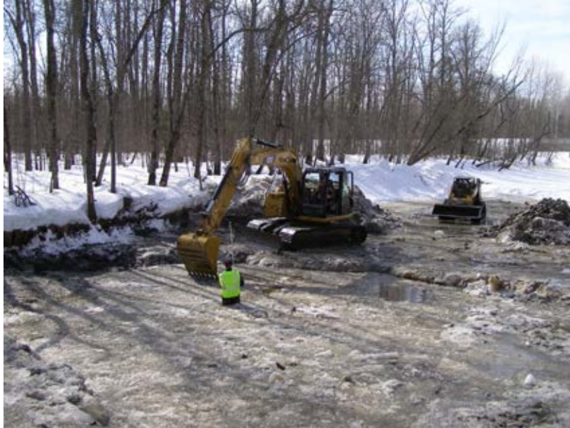
Photo 26-1. Example of riffle construction of Riffle No. 1 during winter 2013. Excavator and skid steer are operating on a frozen Rat Root River. Photo provided by Koochiching County SWCD.
