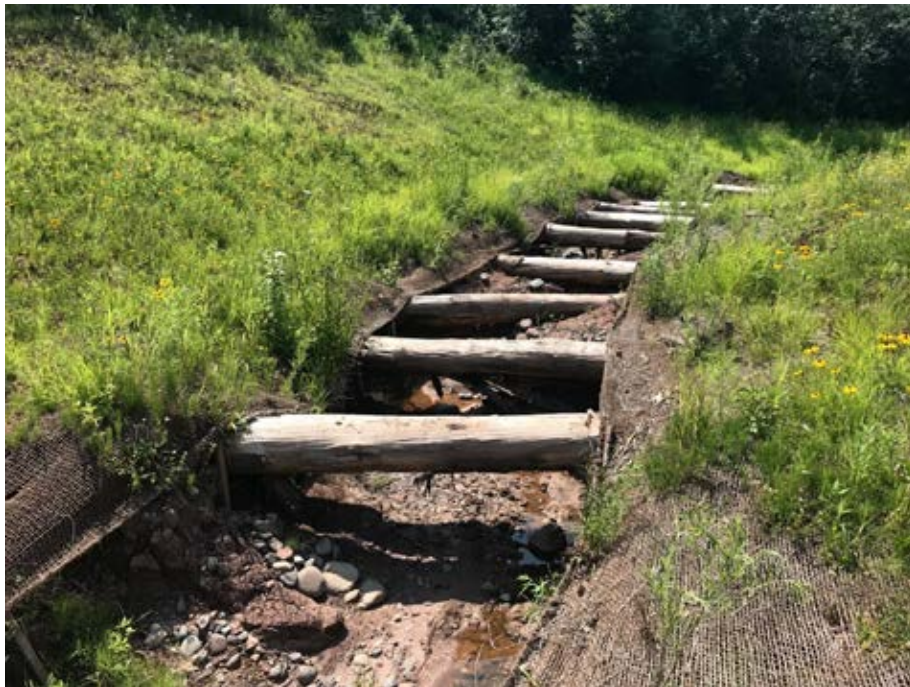
Photo 1-3 Failed log grade control structures within the old dam impoundment. A headcut has advanced throughout the middle section of the project site in an area where sediment deposits were likely the deepest. Photo taken by Mike Majeski on 7/23/2019.
