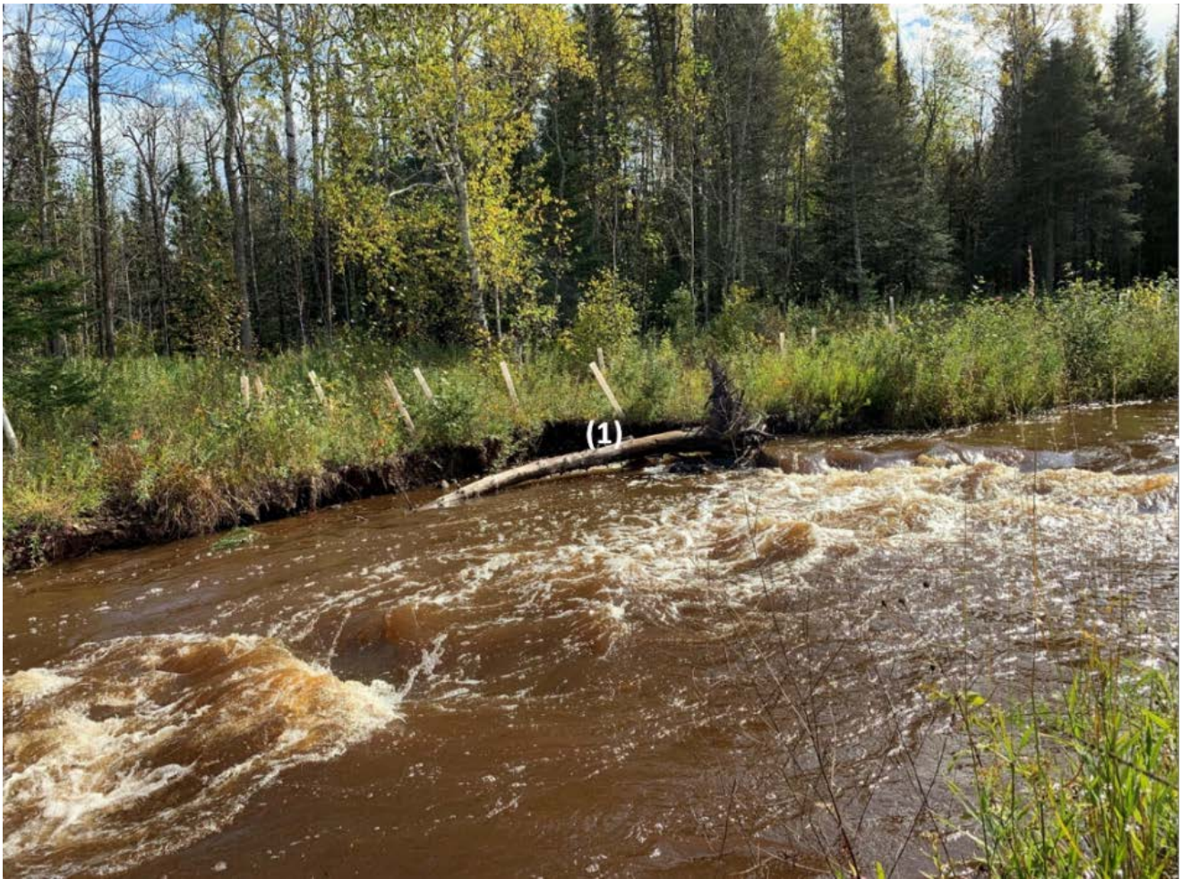
Photo 10-2 – Image of grade control structure (rock riffle) at a period of high (near bankfull) river stage. Note the erosion on the opposite bank, which is likely a product of water deflection from a log (1), which was caught on the structure this past spring. Photograph taken by Kevin Biehn during 10/1/2019 site visit.
