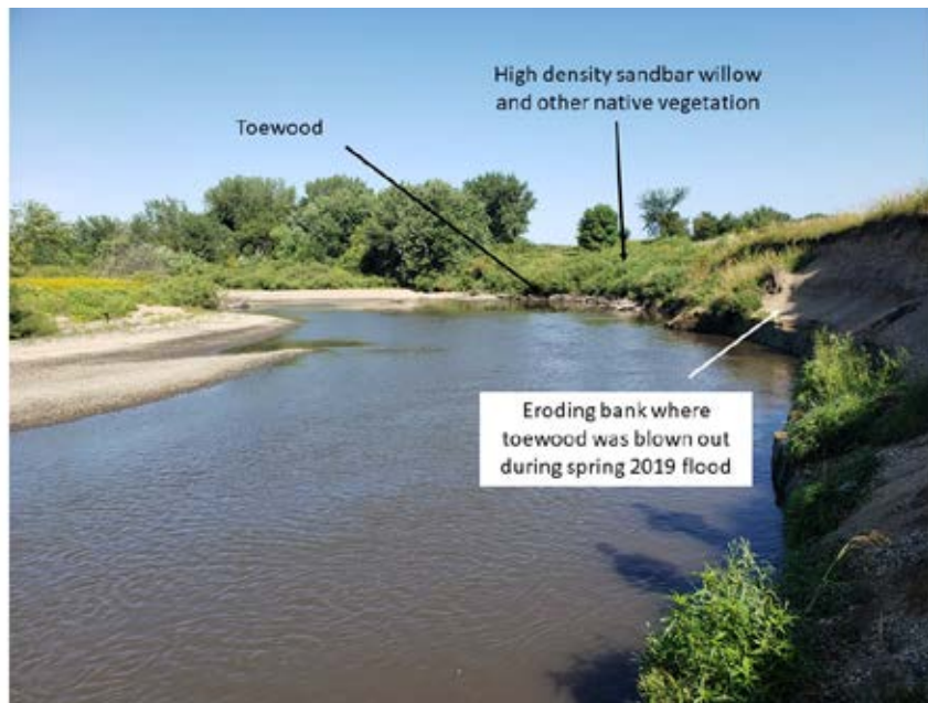
Photo 27-3. Looking upstream at the Downstream Bank (Bank 3). The upstream portion of the bank demonstrates the existing toewood used to stabilize the bank. Above the toewood, sandbar willow have colonized the lower and upper banks. At the top of the bank, primarily smooth brome and other comprise the majority of the cover. Approximately the last 150 feet of toewood blew out during spring 2019 flooding. (Photo taken 8/22/19 by Mark Pranckus, Cardno).
