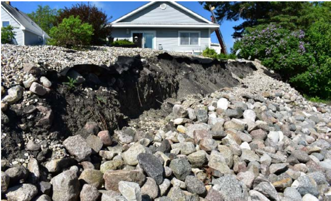
Photo 12-4 View of the disturbance at the top of the streambank which may be signs of a rotational failure or slump. Regrading of this ridge back toward the homes is recommended along with revegetation on the new slope. Photo taken during site visit 06/05/2019.
