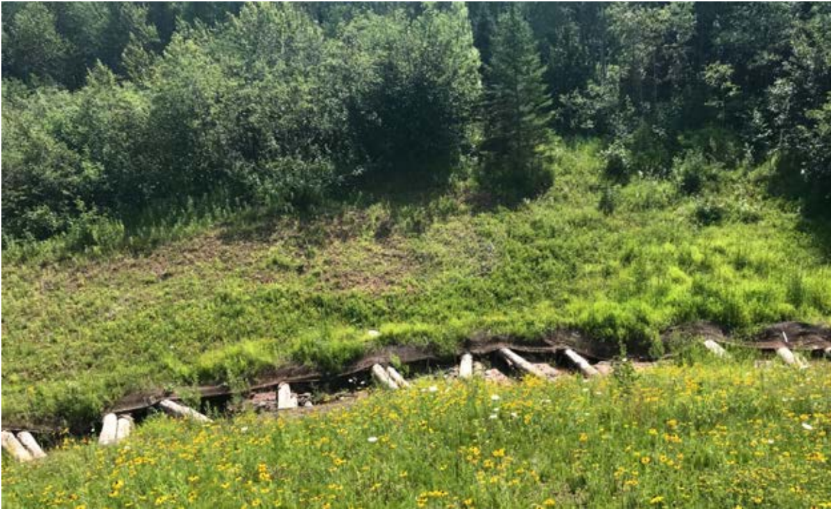
Photo 1-2 Michaelson Dam showing re-graded side slopes with native vegetation establishment. Log grade control structures were installed within the restored stream channel of the unnamed tributary to Deer Creek. Photo taken by Mike Majeski on 7/23/2019.
