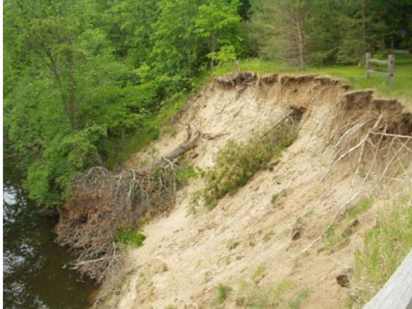
Photo 8-3 Existing steep bank of the West Branch of the Rum River before construction.
