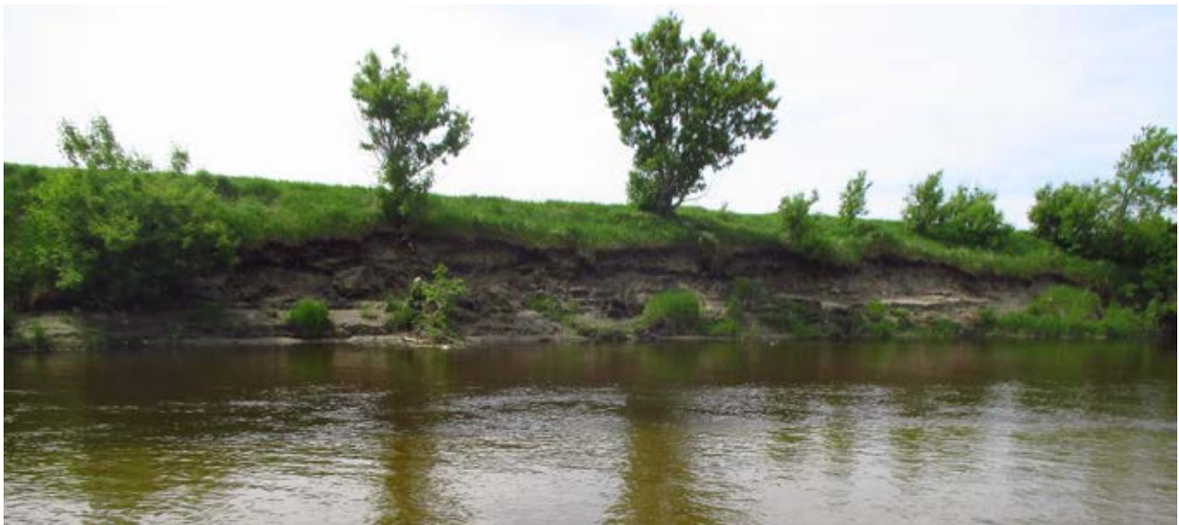
Photo 16-14 Eroding back across from the perched culvert upstream of structure #4 where stabilization and habitat work will be completed with remaining funds. Photo taken during site visit (6/4/2019).
