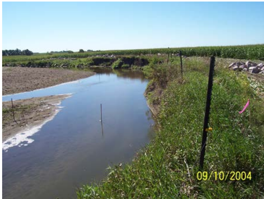
Photo 28-4. Looking downstream near the upstream end of the upstream project area prior to construction in 2014. Note the nearly vertical, severely eroding banks. Rocks used to create the J-hook vanes can be observed along the top of the bank. Photo provided by Scott Ralston (USFWS).
