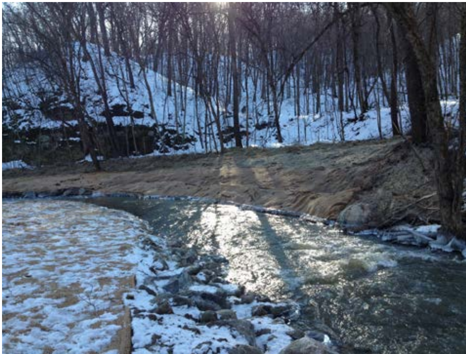
Photo 31-5 Cribwall following construction before vegetation establishment. (Seven Mile Creek County Park, December 2016).
