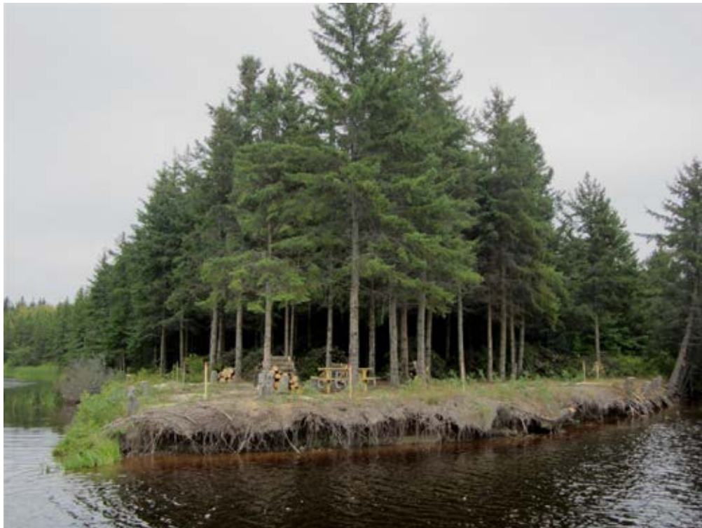
Photo 25-4. Example of the Picnic Site bank stabilization site in 2013 prior to construction. Photo provided by Ed Lombard, Rat Root River Enterprises, LLC.
