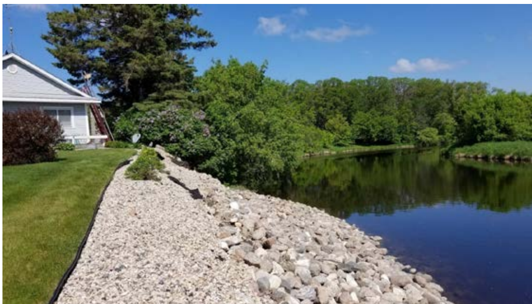
Photo 12-2 Downstream view from 0+50. There is a slope failure present on the upper slope resulting from a freeze-thaw or a quick drop in water level. It is recommended to add biological improvements. Photo taken during site visit 06/05/2019.
