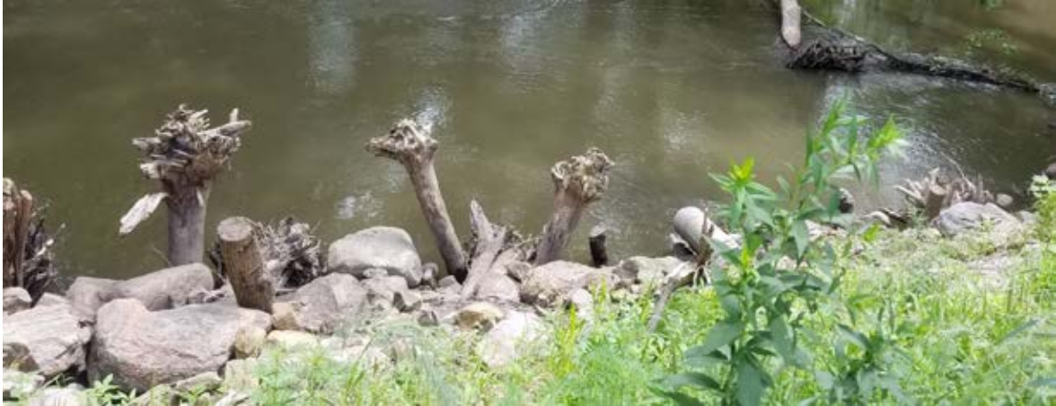
Photo 2-3 View of Adams Washout. Boulders, rootwads and pins holding bank. Photo taken by Ed Matthiesen during site visit (8/13/19).
