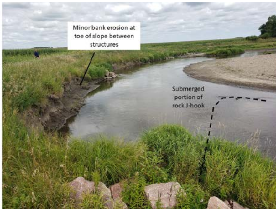
Photo 28-3. Looking upstream at the upstream project area. Minor bank erosion is occurring along the toe between J-hook vanes No. 4 and 5. (Photo taken 8/22/19 by Mark Pranckus, Cardno).
