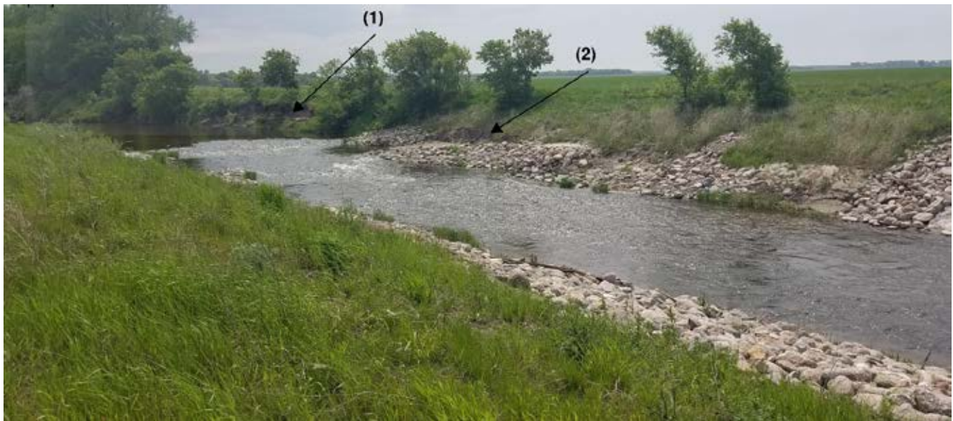
Photo 16-11 Sand Hill River fishway ramp #4 after the original drop structure was modified for fish passage. Upstream of the project area a washout is visible (1). Washout area will be repaired after the culvert connecting the reach to a side channel is addressed. There are also limited bare spots that could be reseeded in the project area (2). Photo taken by Ed Matthiesen during site visit (6/4/2019).
