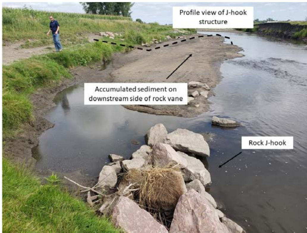
Photo 28-5. Looking upstream at the downstream project area. The two rock J-hook vanes installed in the project area can be seen. A large amount of sediment has accumulated between the structures, which helps to build the bank and protect against erosion. If the upstream vane angle was greater and extended into the channel more, the sediment in the hook of the vane would likely be scoured out, creating pool habitat. (Photo taken 8/22/19 by Mark Pranckus, Cardno).
