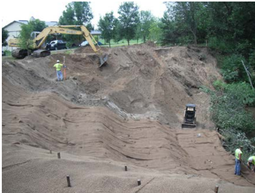
Photo 8-4 Bank resloping and terracing during construction. Seed and erosion control blanket installation is occurring as construction progresses and the anchored trees and brush, and brush fascine are installed at the two of the slope on the river.
