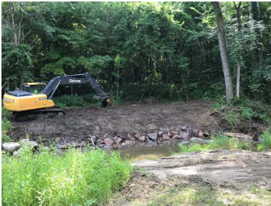
Photo 31-7 Cribwall during reconfiguration repairs. (Seven Mile Creek County Park, photo taken by Mike Majeski at EOR, Inc. August 2019).
