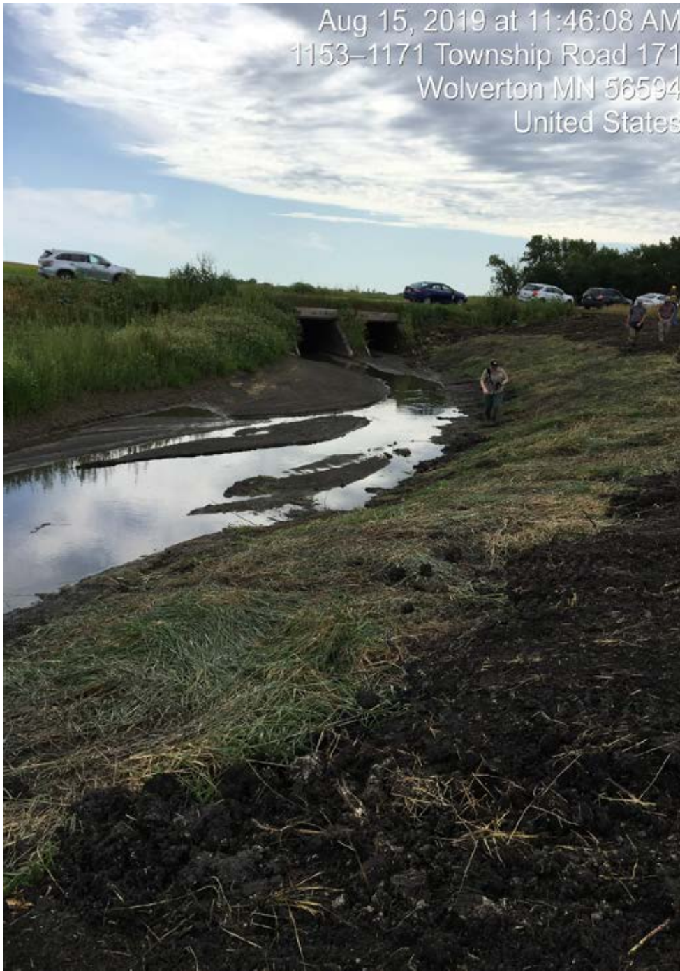
Photo 13-2. Section of stream that has been re-constructed. Photo taken by Anna Varian during site visit (8/15/2019).
