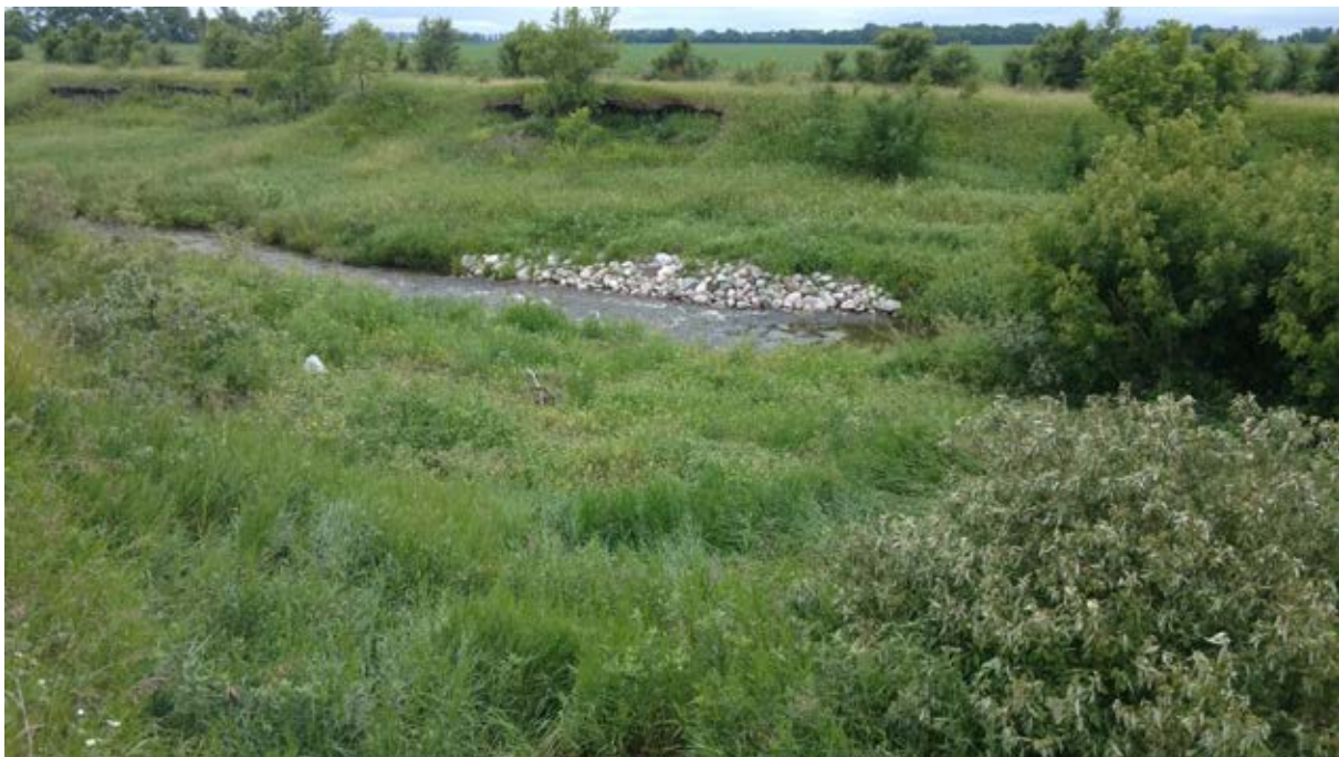
Photo 15-2 View of constructed riffle at project station 91+85. Pre-existing bank slump failures are still visible in the background. Photo taken by others during a post-construction, final inspection (6-29-2017).
