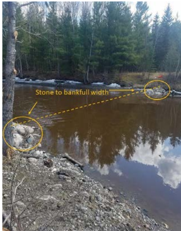
Photo 26-4. Example of a completed constructed riffle. The stone extends to the bankfull width and is throughout the entire channel. Photo provided by Koochiching County SWCD.
