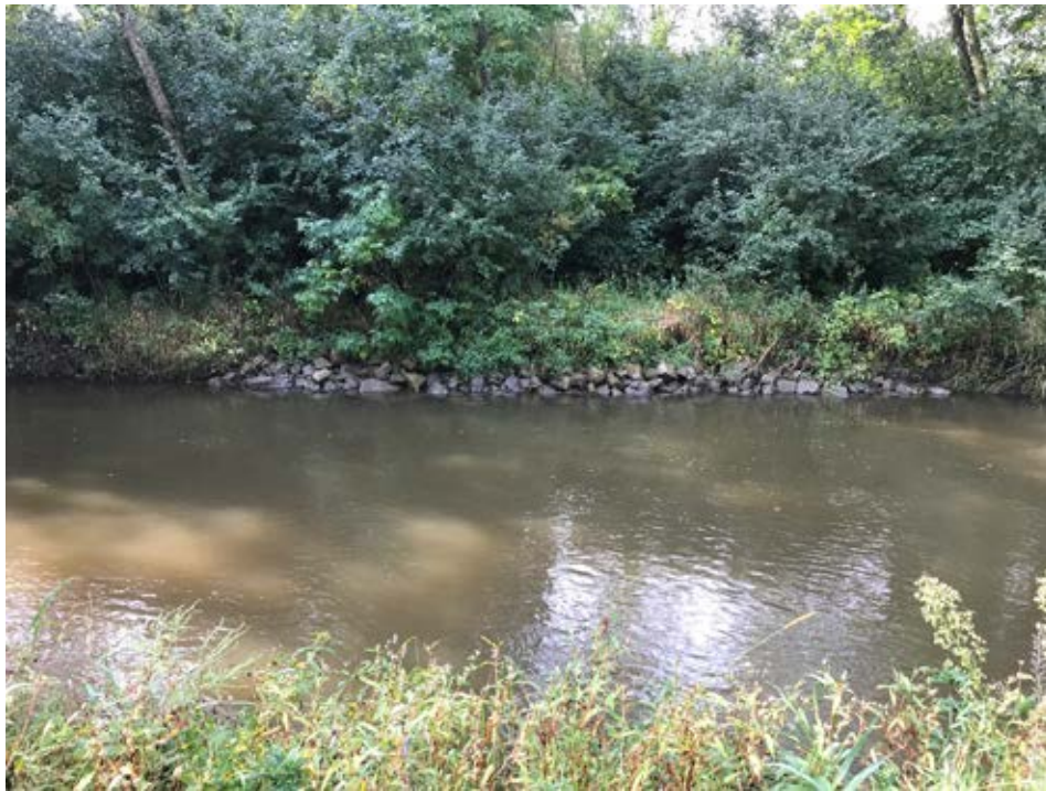
Photo 32-5 Riprap toe installed on the reach 6 project of Wedge Creek. (Wedge Creek – Reach 6, photo taken by Lucius Jonett during site visit 09/20/2019).
