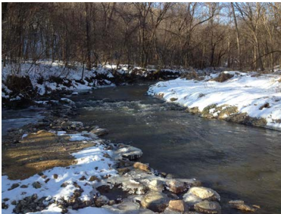
Photo 31-1 Upstream most riffle after original construction. (Seven Mile Creek County Park, December 2016).
