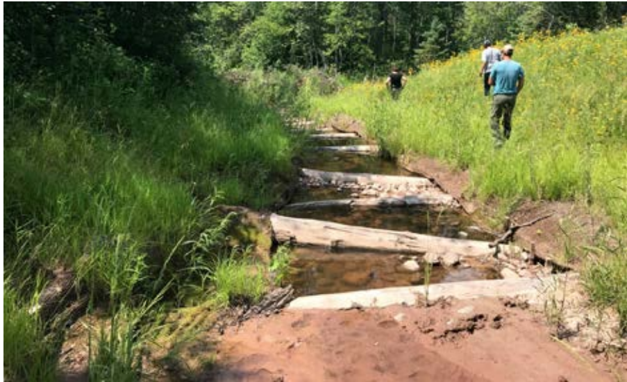
Photo 1-4 Log grade control structures near the confluence with Deer Creek. These structures are intercepting some sediment and are providing small pool habitat for aquatic organisms. Photo taken by Mike Majeski on 7/23/2019.
