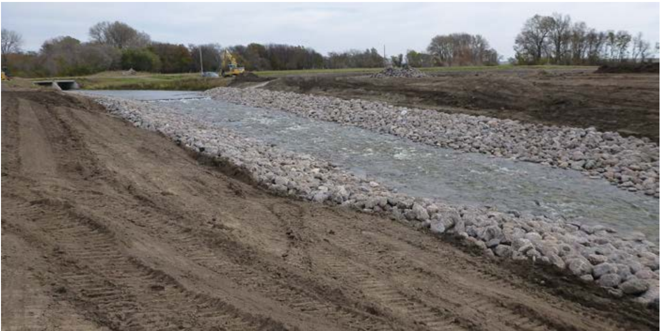
Photo 16-3 Drop structure 4 during construction of fishway. Photo provided by project partners (taken 10/14/2019).
