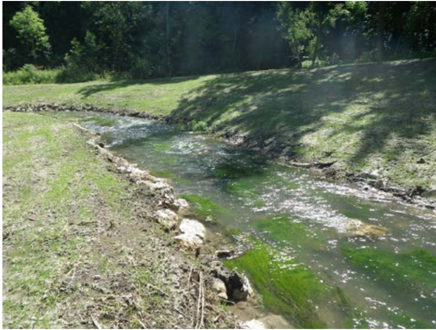
Photo 22-9. Example of Pickwick Creek following construction in 2011. Banks were seeded and straw mulched. The low bank on the left helps to reduce shear stress on the outside bend during high flows. Photo taken August 2011 and provided by MN DNR.
