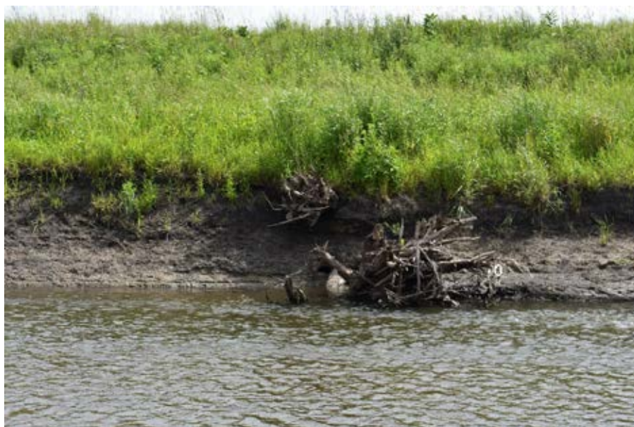
Photo 3-2 View of Elm Creek project showing a single exposed rootwad. Evaluator recommends rock/boulders on both sides of the rootwad near station 7+00 to prevent bank scour behind the rootwad. Photo taken by Ed Matthiesen during site visit (8/13/19).
